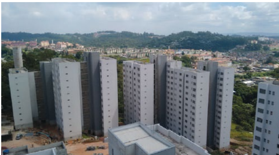
Figure 14: Florestan Fernandes and José María Amaral housing project. Photo: fablablivresp. Source: https://publications.iadb.org/publications/spanish/document/Vivienda_Qu%C3%A9_viene_de_pensar_la_unidad_a_construir_la_ciudad.pdf
